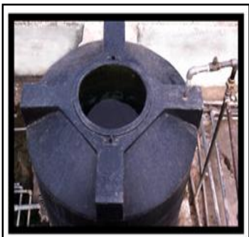
Open overhead tank
